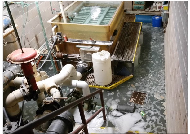
The pool mechanical room experienced a flood on Monday, November 27, when a control valve failed. Another closure came Wednesday, November 29, when a supply valve and pump malfunctioned.
