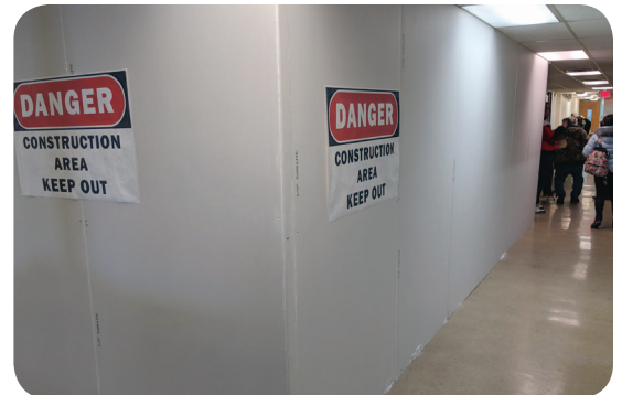
A TEMPORARY WALL HAS BEEN CONSTRUCTED AT THE YMCA AS CREWS WORK TO CREATE THE SYSTEMS CONTROL LITTLE SPARKS CHILD CARE CENTER, NEW PUBLIC RESTROOMS AND A LOBBY/COMMONS AREA NEAR THE WELCOME DESK.
